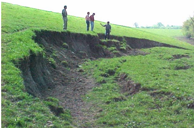
Figure 1: Slide in the Mississippi River levee system
