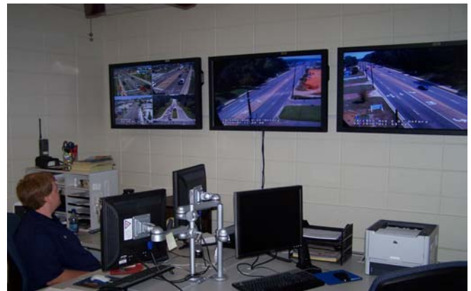
Figure 5: Oxford Police Dispatch/TMC Room
